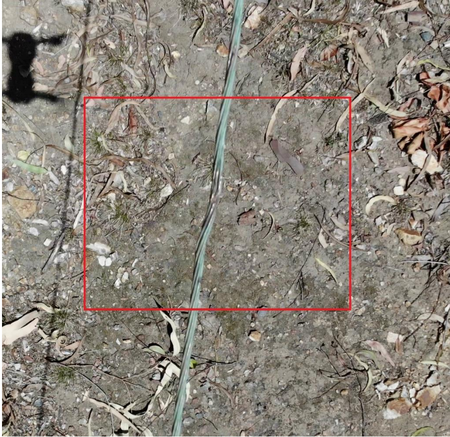
Figure 11 Loss of cross section possibly due to arcing in the test conductor.
