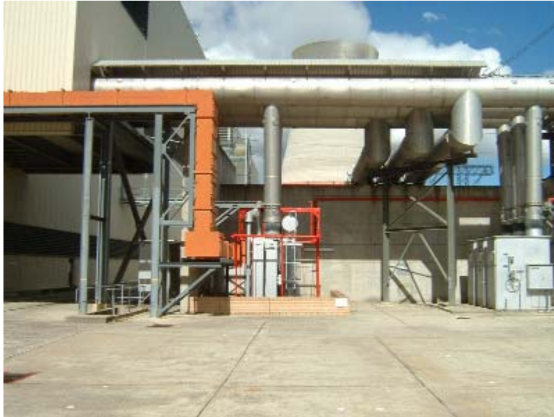
Figure 1. Busbars between a generator, step up transformers and auxiliaries transformers
