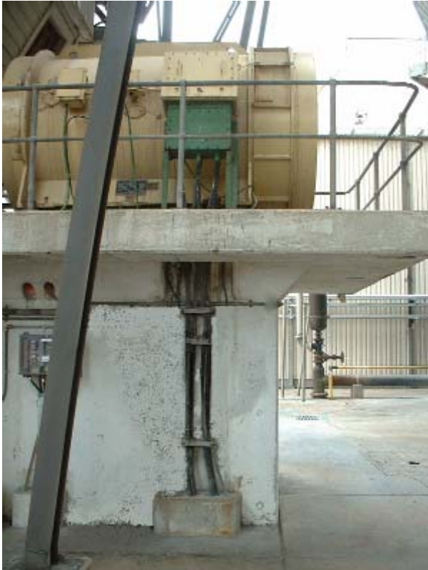
Figure 3. Cabling between switchboard and large motor.
