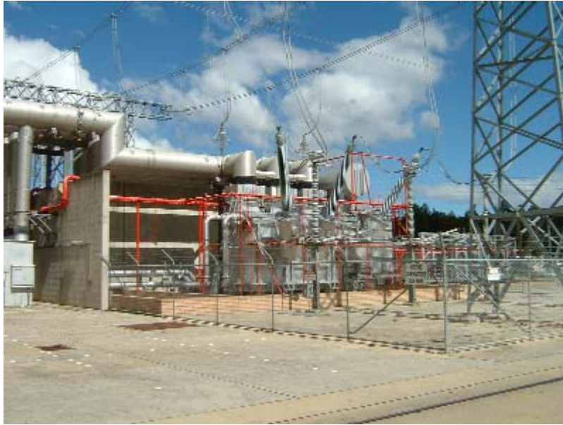
Figure 4. Overhead lines in a generator (step-up) transformer and switchyard area.
