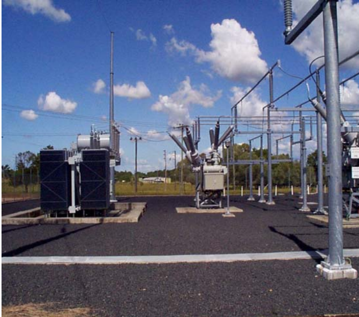
Figure 5. Transformer bay in transmission substation
