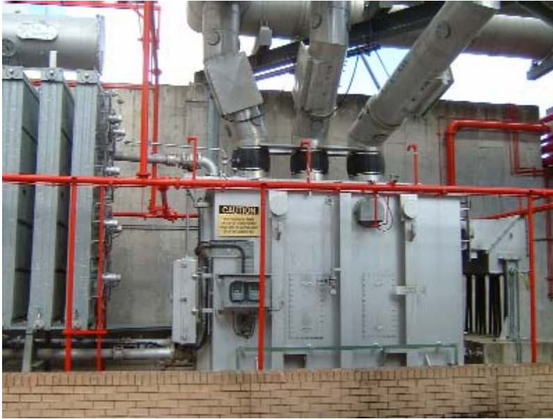
Figure 2. Secondary side of large transformer should be assessed
