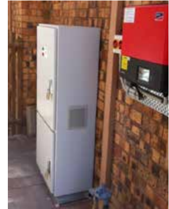
Residential battery storage cubicle with solar inverter in the foreground
