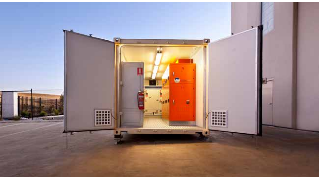
FIGURE 3 400KWH, 100KW LITHIUM POLYMER DEMAND BATTERIES
