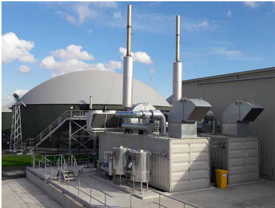
Figure 10 Rewaste Plant at Yarra Valley Water
