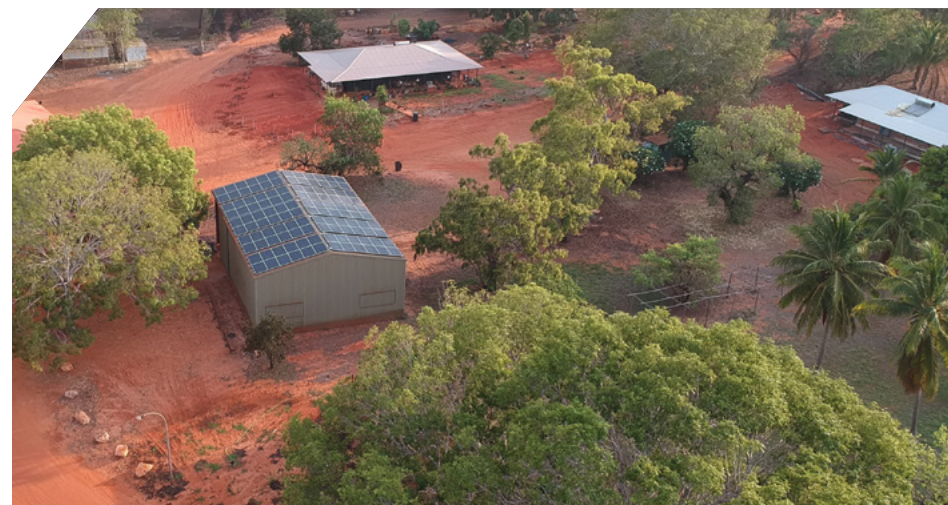
Horizon Power's solar installation at the Lombadina community on the Dampier Peninsula, WA
