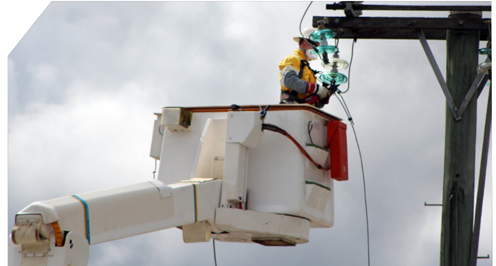
Field Personnel conducting critical works on the Energex and Ergon Energy Networks during the pandemic.
