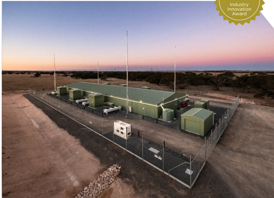
ElectraNet's Dalrymple Battery Energy Storage from Yorke Peninsula, SA
